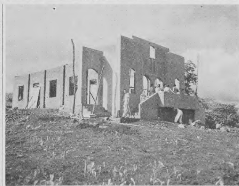
Notice these architectural lines used by Chester Green in designing the new Teapa, Tabasco, Seventh-day Adventist church in the midst of the jungle clearing.
