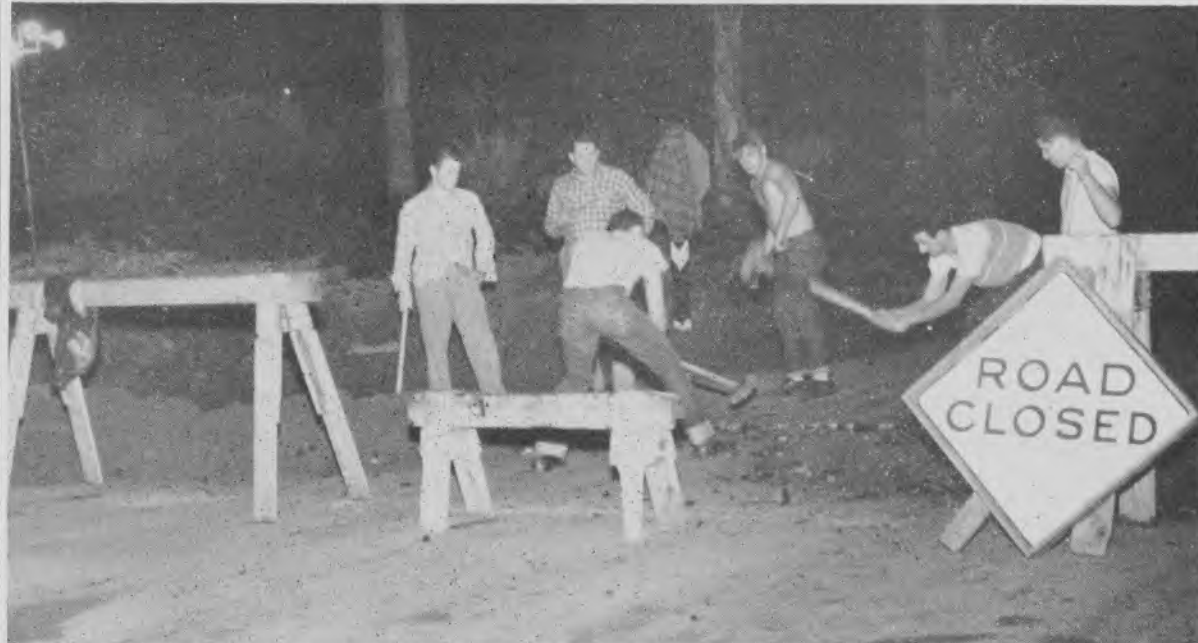
Eager MBK club workers swing into action under portable floodlights to make short work of a ditch-digging project for which the club submitted the low bid. The treasury of the men's organization, now $200 ahead, received a check from the LSC business department Thursday evening. Men on the scene of action at picture time are Robert Nelson, Hugh Love (dean of men), Warren Fish, Jack Osborn, Duane Longfellow, and Fred Paap.
