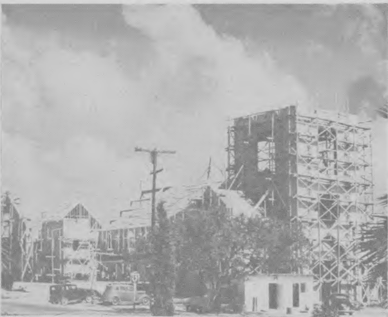
CHURCH ERECTED: Built in late 1947, the La Sierra college church seats 2,200 in the main auditorium. Shown is an old Criterion cut of the structure as it was in the process of construction.
