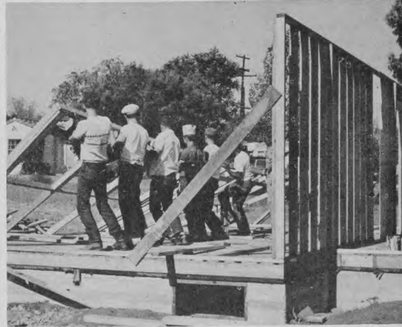
HEAVE-HO: As part of their project in carpentry and construction, students are building a $12,000 house near the college grounds. Actual on-the-job experience is gained in ironing out construction problems. Here, students raise one side of a wall as the outer sections of the new house begin taking shape.
