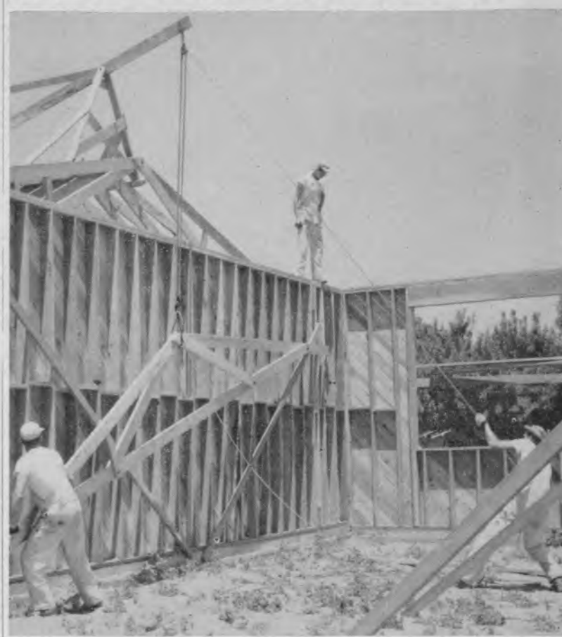
LSC students raise rafters and pound nails on new academy construction. Here John Kerbs, Willis Wilcox, and J. C. Gentry put roof timbers into place. PHOTOS BY TALLANT
