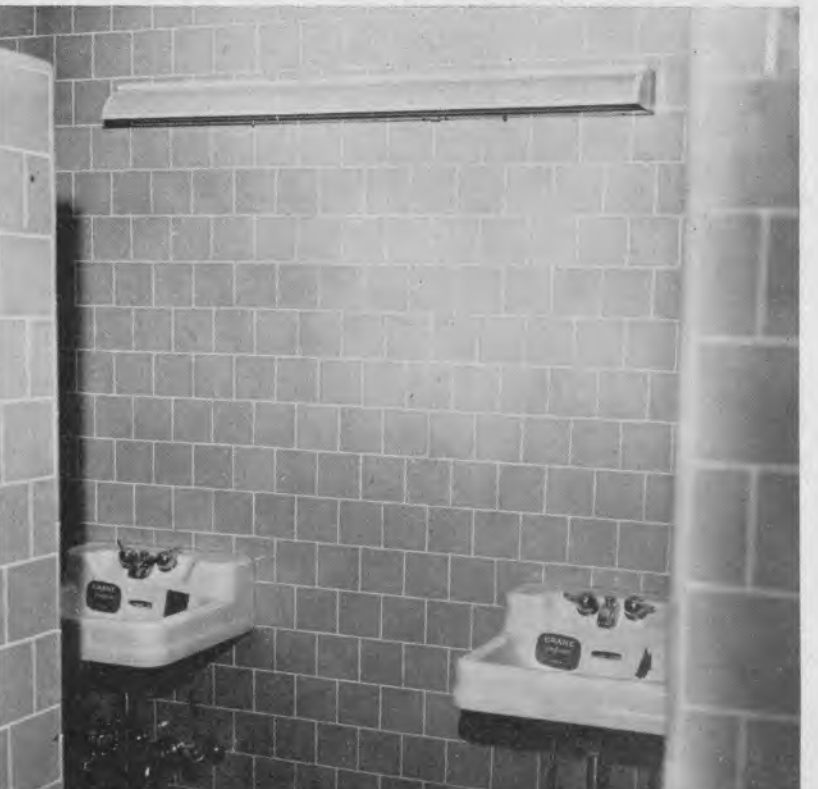
Completely rebuilt with tiled walls and floors and with new fixtures, these Calkins bathrooms will look new for years to come.
