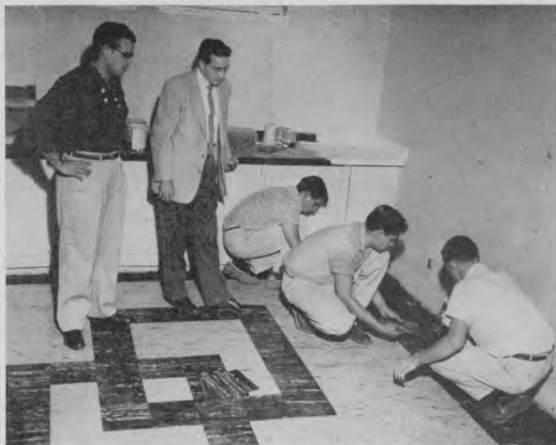
ASB HEADQUARTER'S RENOVATION continued off and on during the past summer and on into last week. Here ASB proxy Sterling Ryerson and Graduate Manager Lawrence Mobley note, on the side-lines, the finishing touches put on the METEOR floor by METEOR Editor Edmond Phillips and his staff.
