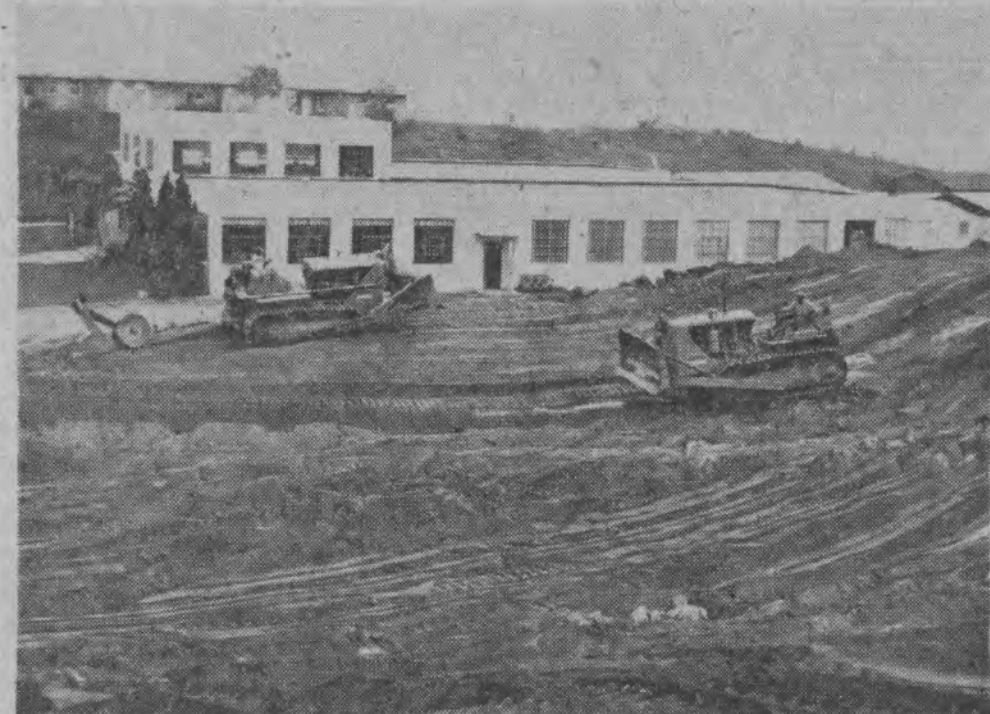
A small-sized mountain behind the Home Economics building began its final death struggle as earth moving equipment carted soil and granite away for use on the new highway being constructed in front of the college. Who said Giants were a thing of the past?
