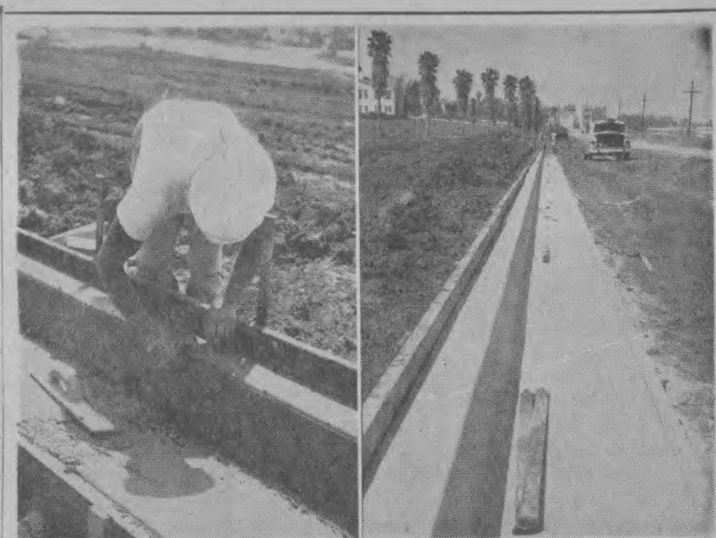
It may be hard to believe but progress is being made on the new highway. Some 40 working days were lost during the rainy spell, officials report. If the thoroughfare is not completed within 24 days, the County will receive money from the company building the road instead of giving it out, it was further stated.
