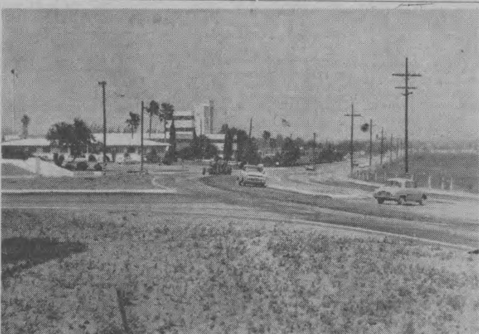
The new highway under construction as seen from the College service station. Rains have hindered work, and subsequent hot weather and wind have stirred up dust storms to the dislike of students and faculty.
