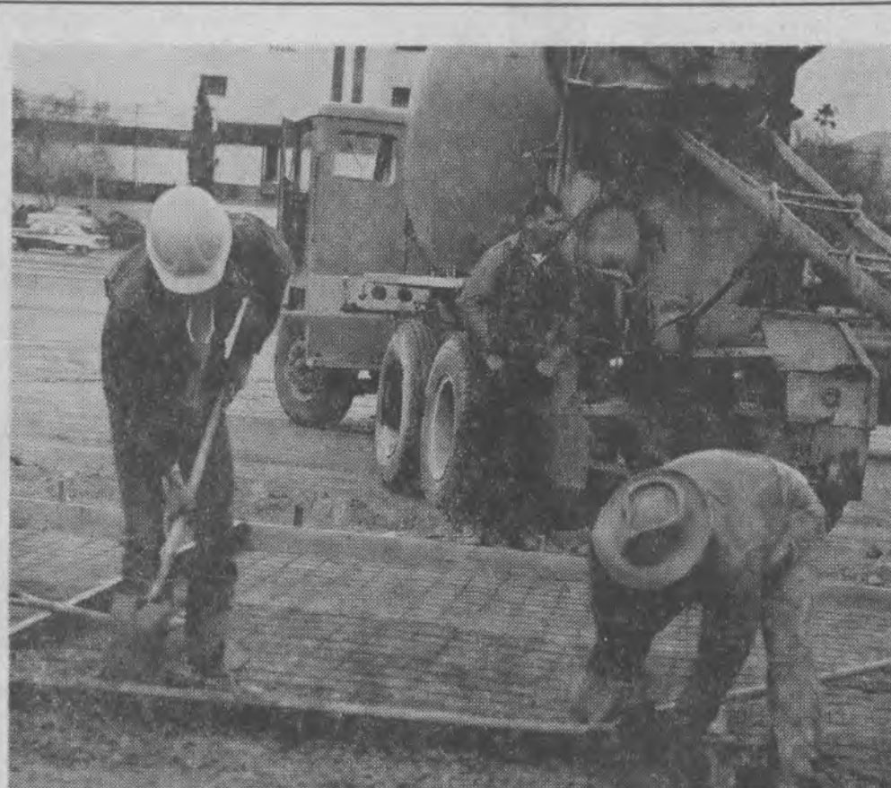
POURING CEMENT—Workmen are readying the foundation for the new College Market in preparation for raising the tilt-up concrete walls.
