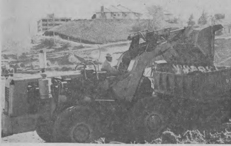
UNDER CONSTRUCTION—Work has now begun on the $404,000 home economics building. Construction is slated to be completed in early 1968. In the background can be seen the new high-rise men's dormitory.
