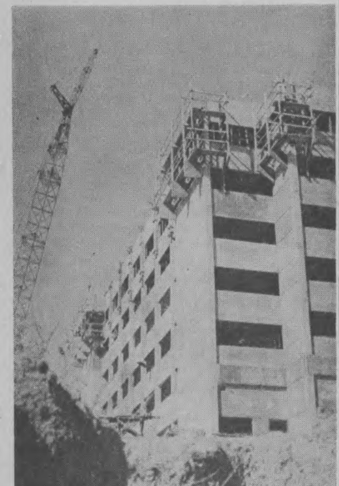
REACH FOR THE SKY — The seventh and last floor of the new men's residence hall is now being poured. Final completion for the dorm is set for August 1, 1967.
