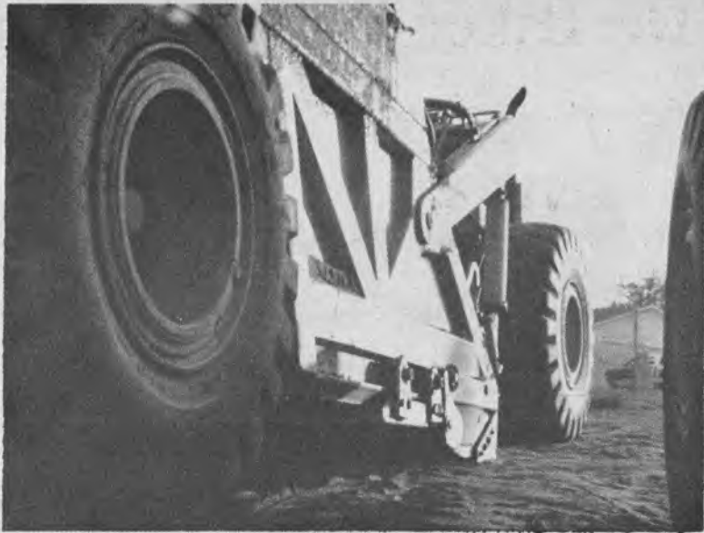
CAMPUS INVASION--Since Christmas vacation earth-moving equipment has been noisily removing the hill where the library will soon be constructed.
