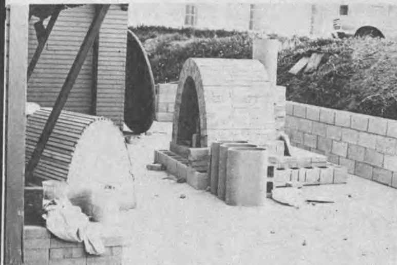
Shown above is a sketch of the inside of the kiln now being built by members of LLU's Art Department. Below is a photograph of the kiln as it appears at present. The project is located behind the Art building.
