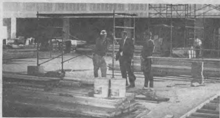
HAL WILLIAMS (center) of the Alumni Association, discusses construction progress with a workman and a member of the P. E. department staff. The gymnasium is scheduled for student use by early March.
