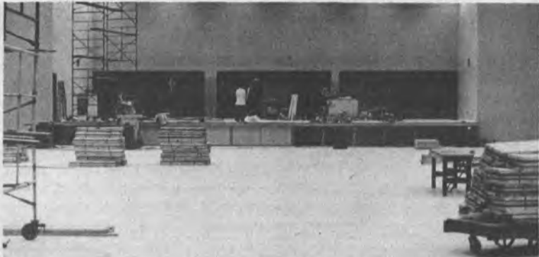
An interior view of the new Alumni Pavilion. Photo was taken Thursday morning; the floor is expected to be installed in time for the first program in the building tomorrow night.
