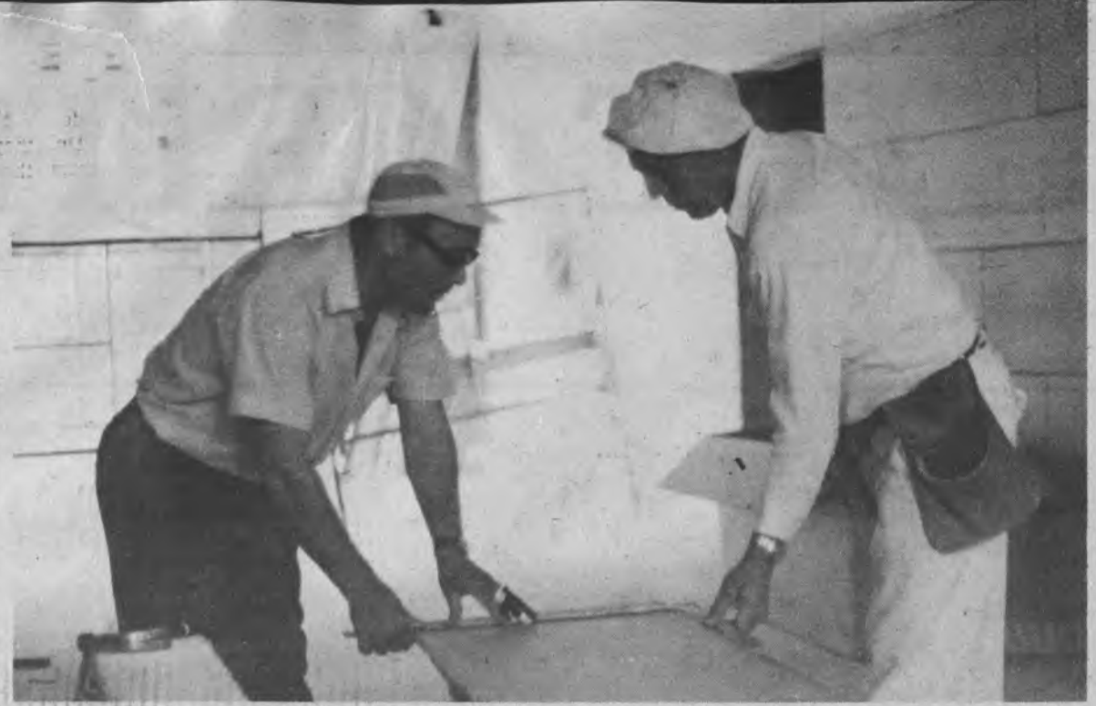
Work nears completion on new offices and classrooms in the administration building.
