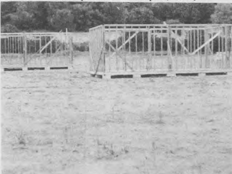
Construction students are building sheds while they await city permits to begin work on a new house.
