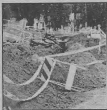
Long trench is being dug by construction crew to extend from central power vault to Palmer Hall
