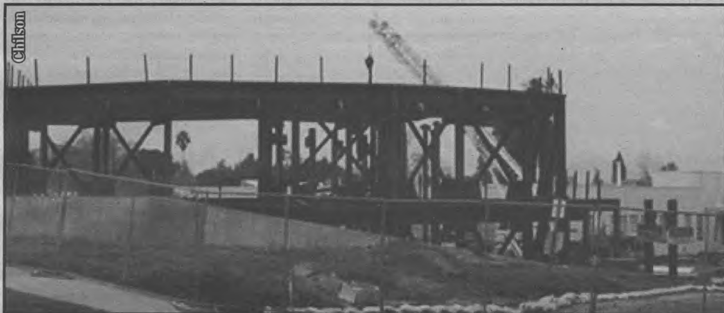
Construction continues on the Thaine B. Price Science Complex. The project is scheduled for completion in spring of 2006.
