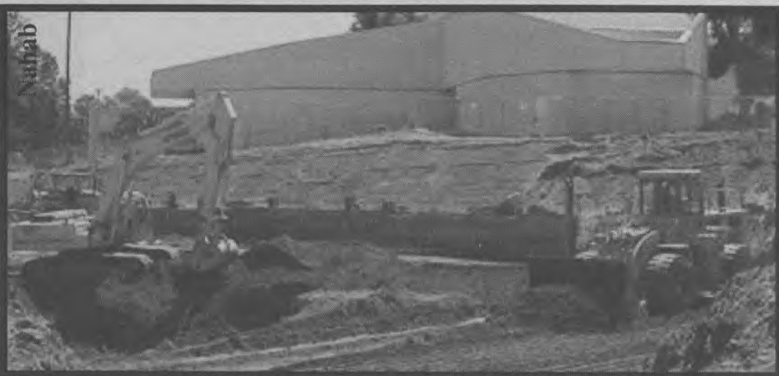
Bulldozers at the construction site of the Thaine B. Price Science Complex clear the way for the building's foundation.
