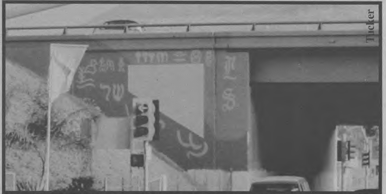
Workers have begun placing the mural on the Pierce St. overpass, adding a splash of color to the cold concrete.
